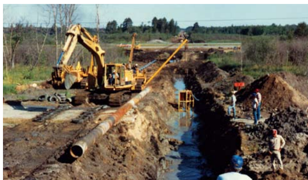
In 1983 and again in 1985, the MPL system expanded by constructing "loops." These new sections and extensions added nearly 100 miles of pipeline to the system.
