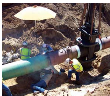
2008 – The final weld by a crew from the same company that helped expand the MPL in 1983.
